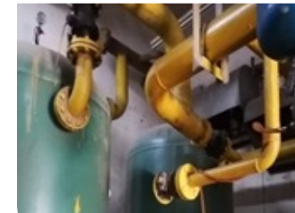
Reconfiguration of compressed air pipe system in China resulting in an estimated energy savings of 945,000 kWh/year.
